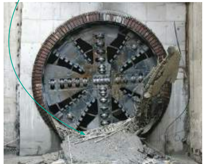
Structure of concrete & FRP bars crushed by TBM
